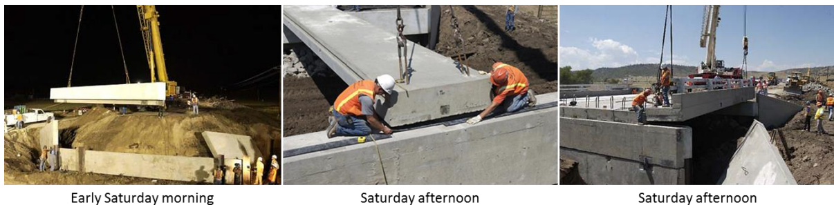
Figure 3 Bridge made in ABC technology on the State Highway 86 over Mitchell Gulch in Colorado in 2002 ( http://utcdb.fiu.edu/bridgeitem?id=185# ).
