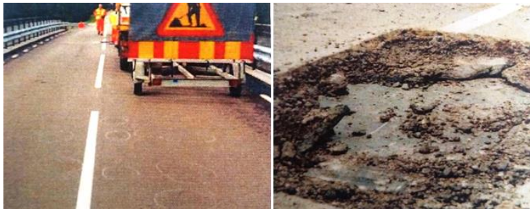
Figure 4 Typical delamination of damage of asphalt layer placed on the concrete bridge plate (Westergren 1999).
