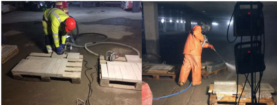
Figure 3-12 Sample preparation at contractor. Grinding on the left and water jetting on the right.
