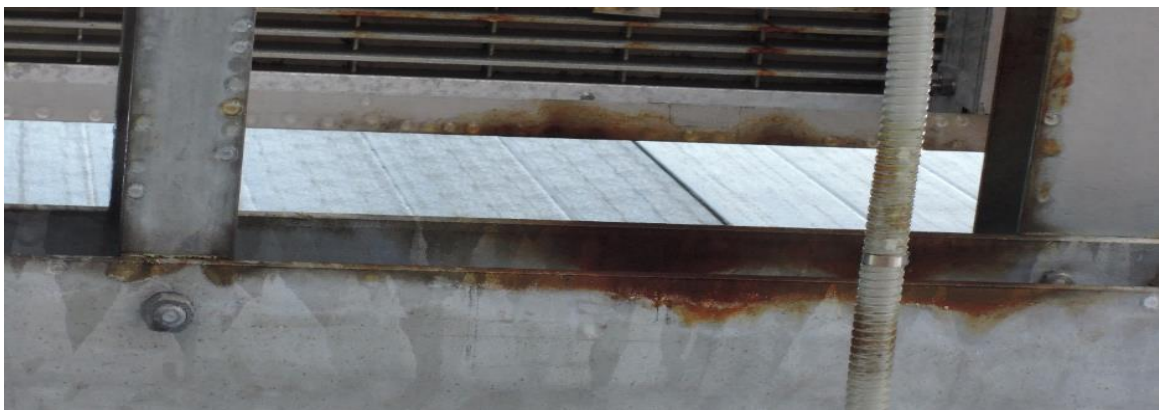
Figure 16. Discoloration from extraneous rust.
