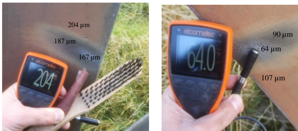
Figure 10. Coating thickness measurements of HDG steel of a 48 year old power pylon placed nearby the E4 freeway in the Stockholm area. To the left: leg furthest away from the traffic, To the right: leg closest to the traffic. Loose corrosion products were scraped using a steel wire brush to produce the blackish surface, further treatment with a 100 grit paper produced a surface with metallic sheen equivalent to a St 3 surface according to ISO 8501-1. Different treatments produce significantly different thickness measurements. It is also noteworthy that the thickness was almost double on the leg furthest to the freeway, in other words, film thickness can be very local. Varying film thickness can be differences from the HDG process or local variations in corrosivity.
