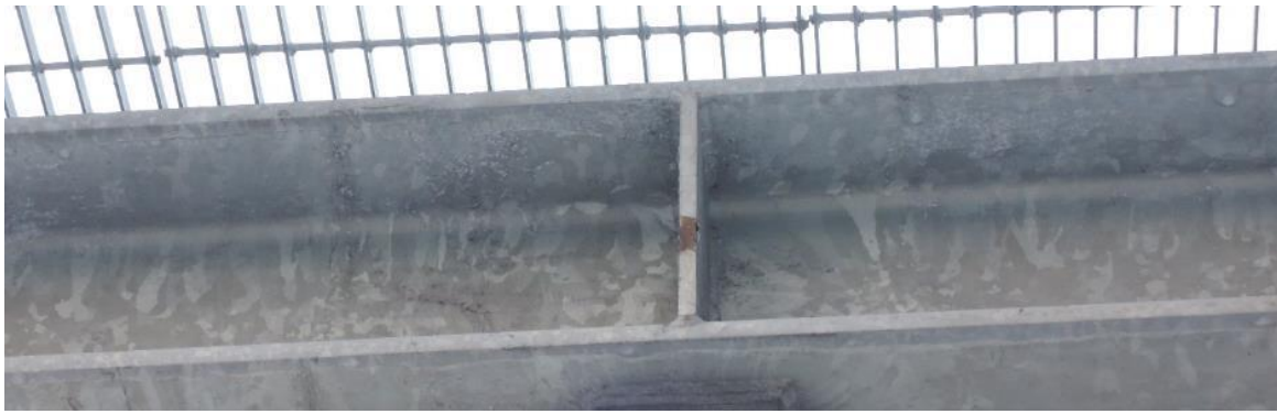
Figure 15. Damage in the HDG coating down to the steel substrate. The damage was located in a position that makes the cause likely to be flaking due to mechanical damage during transportation or structure assembly.
