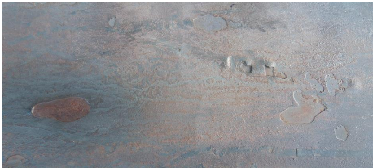
Figure 14. Spot-wise delamination and areas with low zinc thickness. This damage has probably come from the HDG process.
