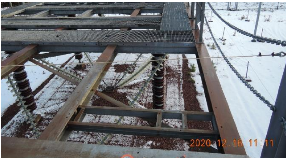
Figure 12. Overview of the transformer platform that was inspected. Generally no signs of critical corrosion damage were found. The main I-beams have developed alloy corrosion.
