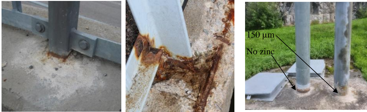
Figure 7. To the left: a HDG railing post cast into concrete about two years after installation, the railing post was found to be in electrical contact with the cast-in rebars. In the middle: a painted railing post with galvanic corrosion between the post and the cast-in rebars. To the right. A concrete slab with two protruding ventilation pipes in HDG steel. The left pipe showed red rust at the interface between concrete and steel. The right pipe showed no corrosion at the concrete steel interface. It is probable that the left pipe is electrically connected to the rebars and the right pipe is not. Electrical contact measurement of this particular installation could have avoided this type of corrosion damage.
