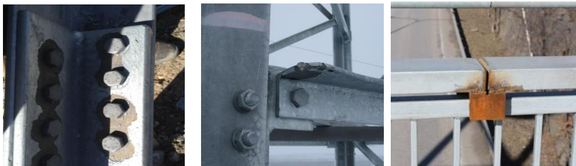
Figure 6. To the left: damage from assembly and inferior zinc adhesion to the steel, the damage may have been avoided with use of proper washers. In the middle: damage from transport, can be avoided with adequate care during handling. To the right: a damage from welding after the galvanization process.
