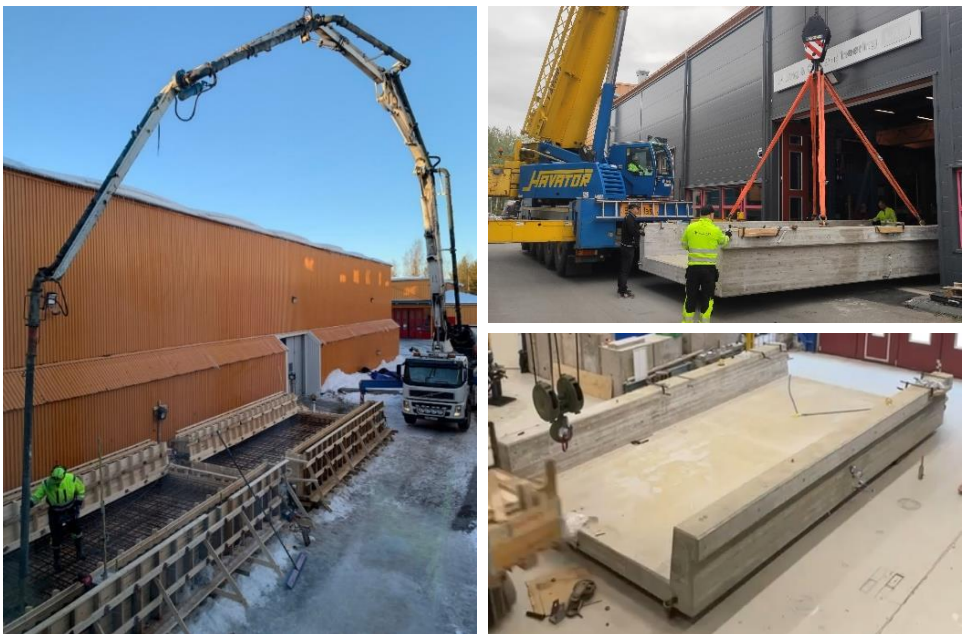
Figure 20: Casting Day for the trough bridges (left), transportation of TB1 (right, top), TB1 inside the laboratory (right, bottom).
