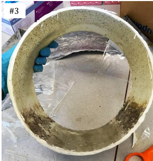
Figure 3. FRP CIPP-liner installed at 2010.
