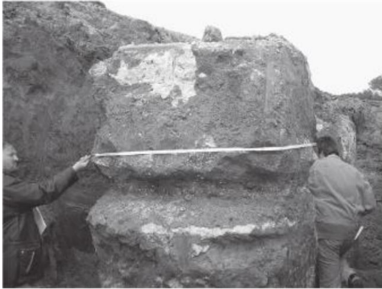
Figure 6 Diameter quality control of jet grout column by excavation (Croce, et al., 2014)
